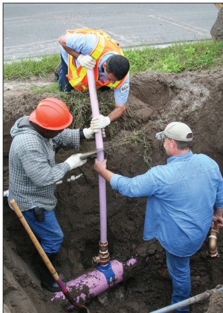
Purple pipes distinguish reclaimed water lines that serve 15,000 customers. The division has one of the largest residential reclaimed water systems in the country.
